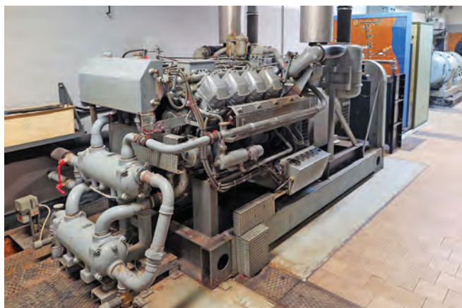
Generator within the Stevns Fort
